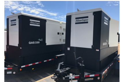
Portable & Standby Generators
